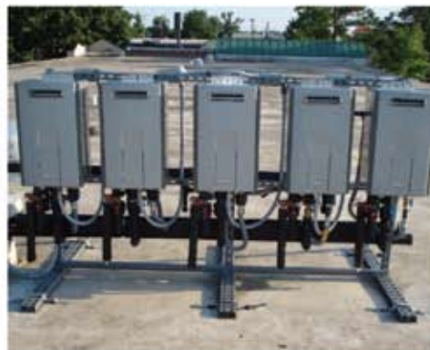
At this 40-room hotel, exterior units are mounted on the rooftop with no additional venting. Hotel owners have experienced 50 percent reduction in therms per occupied room.
