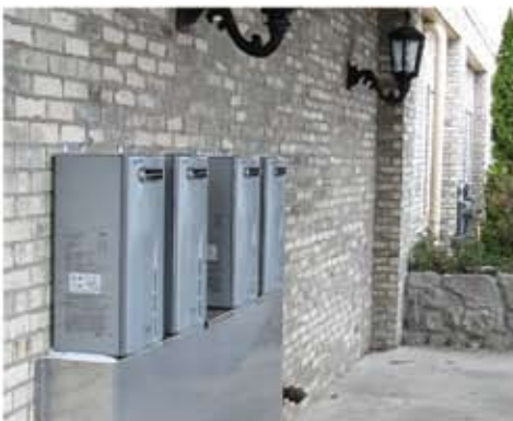
Full service restaurant gains extra mechanical room square footage for additional storage plus redundancy by installing multiple units on the exterior wall.
